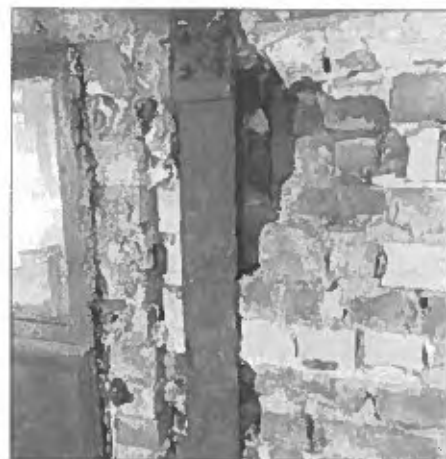
Corrosion found on the rear brickwork face of the building
