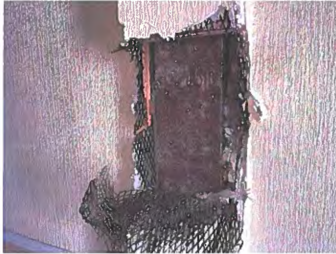
Figure 2.0 Interior Dry Area Corrosion
