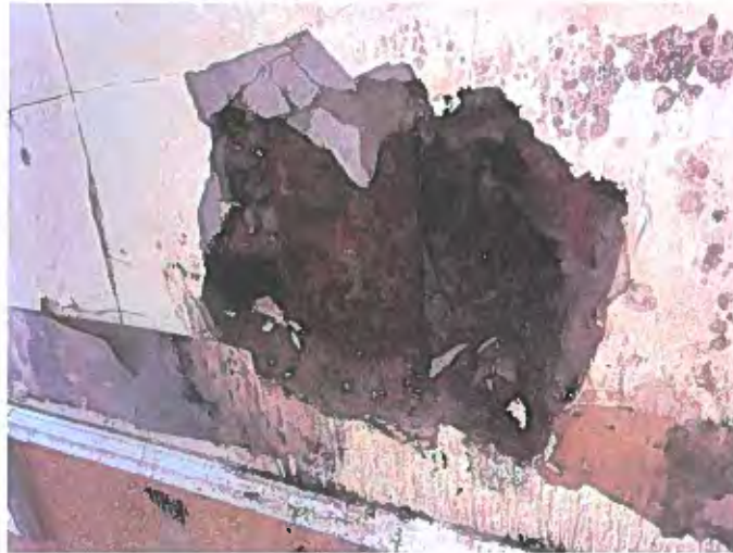
Figure 3.0 Interior Wet Area Corrosion
