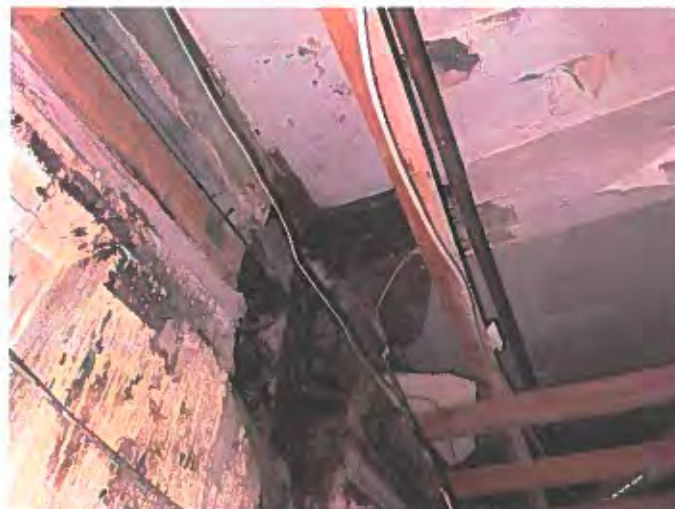
Figure 4.0 Façade Steelwork Corrosion
