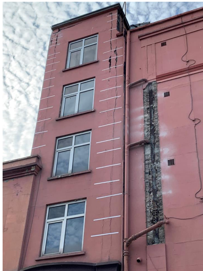
Figure 2 – Images following removal of loose plaster and temporary strapping of existing walls taken in July 2020.
