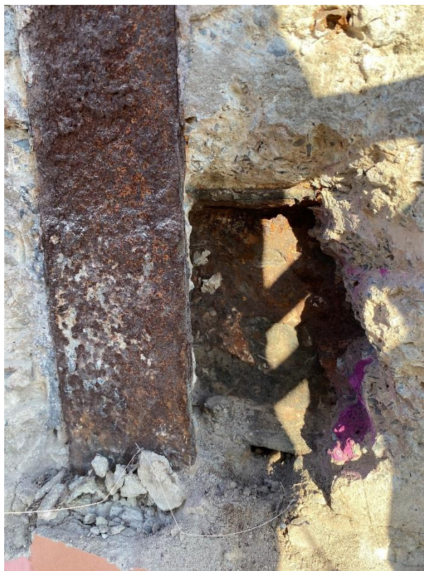
Photo 8 – Crosby Street Beam to Column Connection. Column and incoming beam indicate signs of corrosion and de-lamination.
