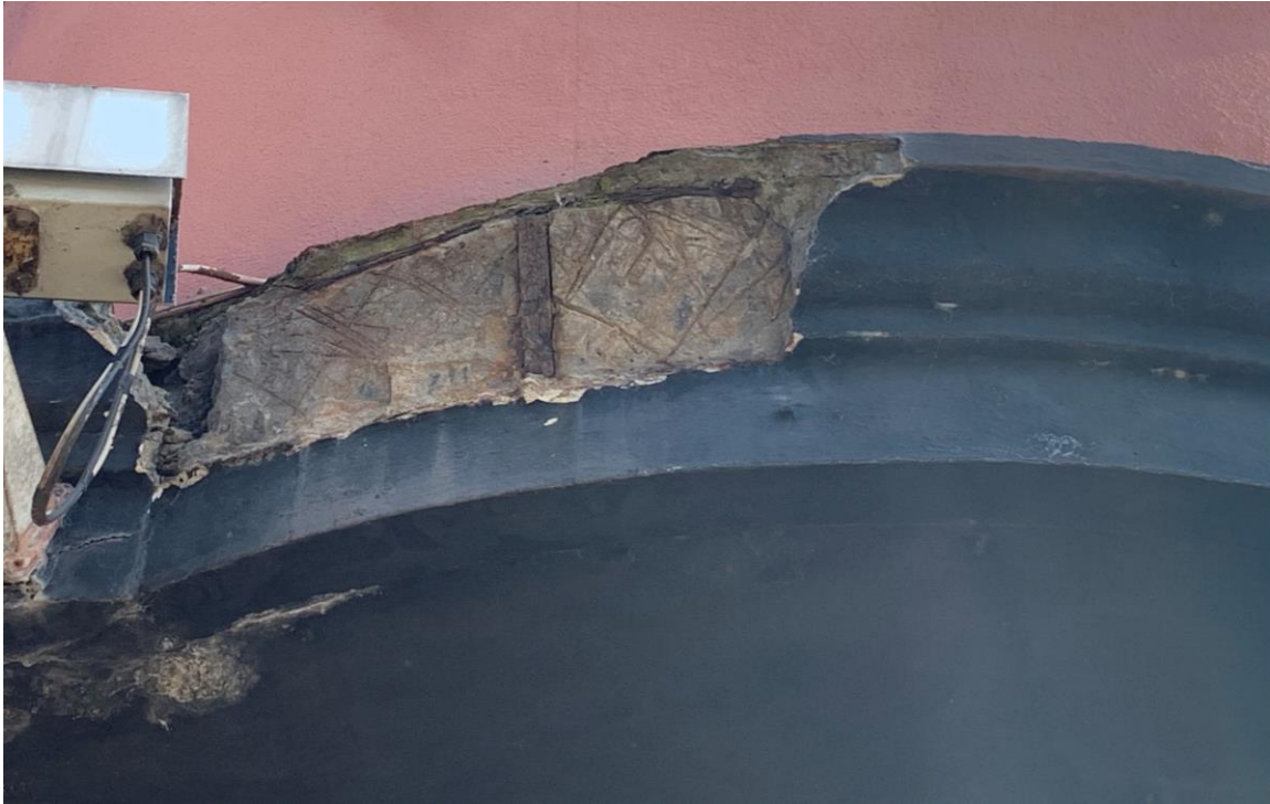
Photo 5 – First floor curved steel beam at corner of Crosby Street and Quay Street. Corrosion and de-lamination of steel top flange is present.
