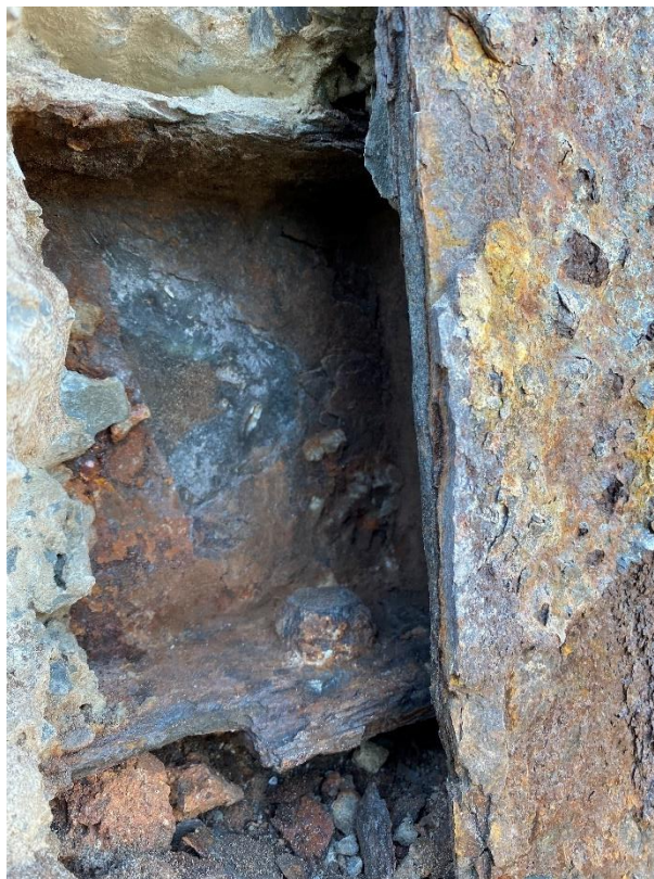
Photo 2 – Crosby Street Column flange with severe section loss and de-lamination of incoming steel beam.
