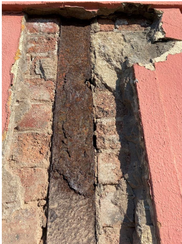
Photo 6 – Quay Street Column showing the typical relationship with the external solid brick wall. The photo indicates de-lamination of the steel flange.
