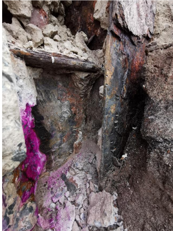
Photo 3 – Quay Street Column Beam to Column Connection at 1 st Floor level. Severe section loss and de-lamination of column flange evident.
