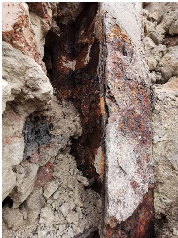
Photo 4 – Photo of column flange on Crosby Street Elevation. Significant de-lamination of column flange.
